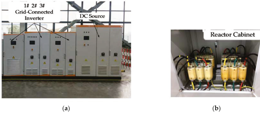
Figure 20. Experimental platform: (a) Three grid-connected inverter and DC source; (b) reactor cabinet to simulate the grid impedance.
