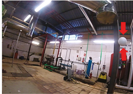
Figure 3. Sphere located in a pillar of the machine room (attached by a neodymium magnet).
