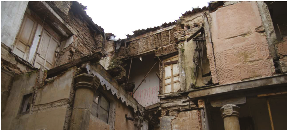
Figure 8. Main cloister; detail of a collapsed wooden floor due to the rotting of the beams.
