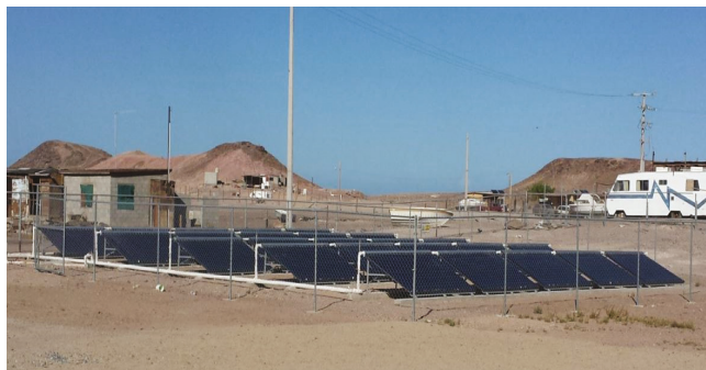
Figure 1. Evacuated tube solar collector field with a bottom parabolic reflector.
