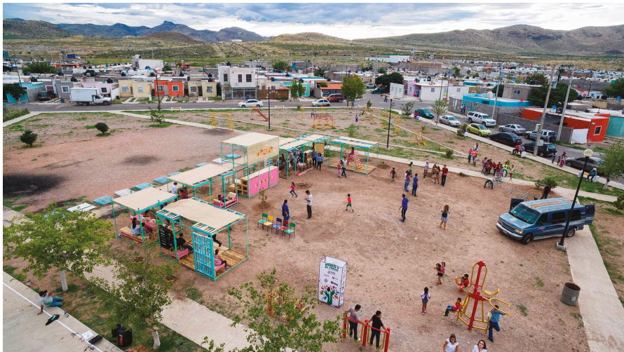
Figure 3. The 'Hands on to my park' project under construction, July 2017. Photograph: DELFOZ, Enrique Portillo.
