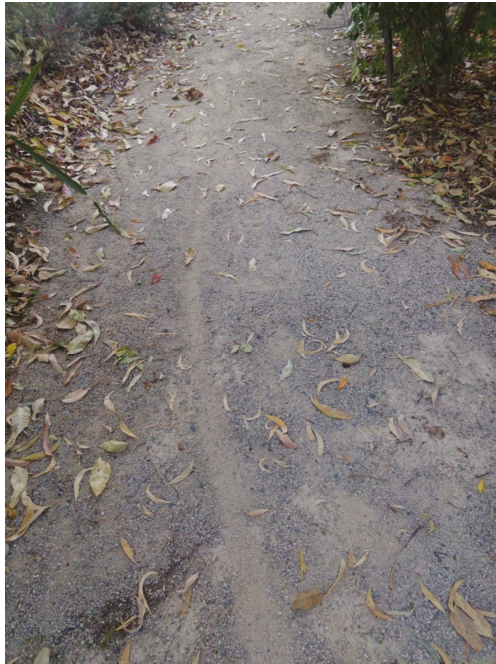
Figure 5. Loose gravel path.
