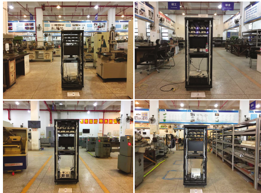
Figure 9. The location of the wireless sensor nodes in the practical industrial scenario.
