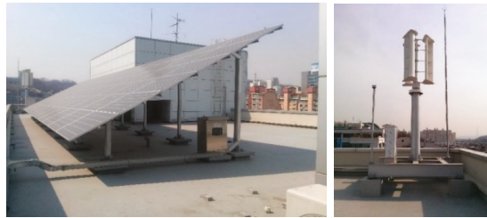
Figure 2. PV and WT system at the Guri office.
