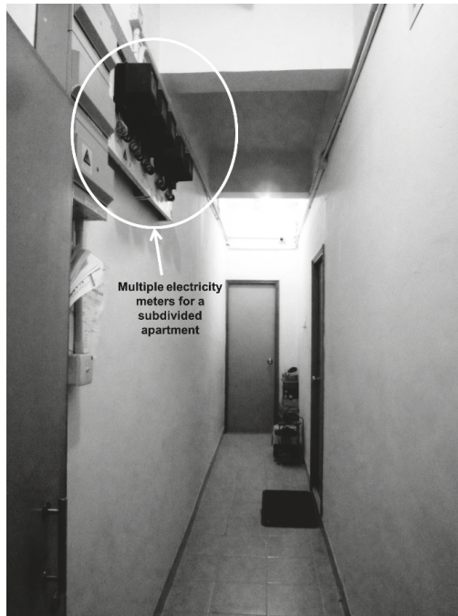
Figure 4. Multiple electricity meters as a signal of flat subdivision.
