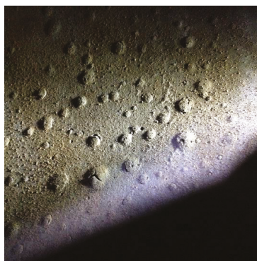
Figure 1. Blistering in internal surface.
