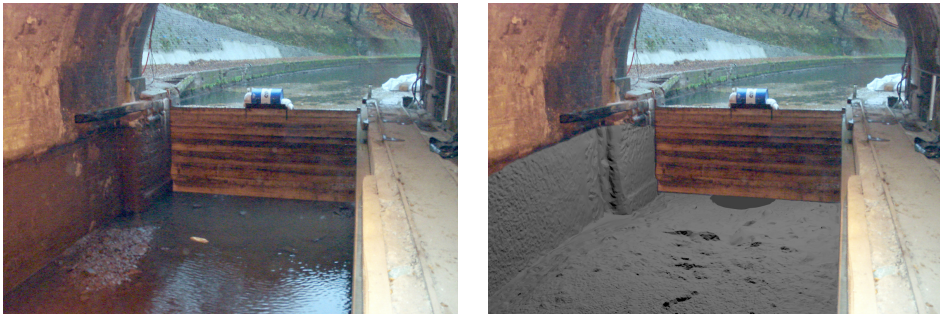
Figure 11. (Left) Photograph on the northern tunnel entry, during its emptying for maintenance in 2009 (source: Voies Navigables de France (VNF) archives); (Right) Visualization of the MSS denoised model (in grey) superimposed on the image. The orientation is done manually, thanks to the masonry block and the cofferdam grooves, which are visible in the model.
