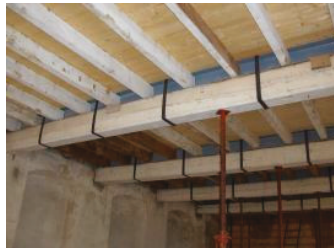
Figure 19. Reinforcement of a timber beam using a stainless steel H-shaped beam applied on the compressed area.
