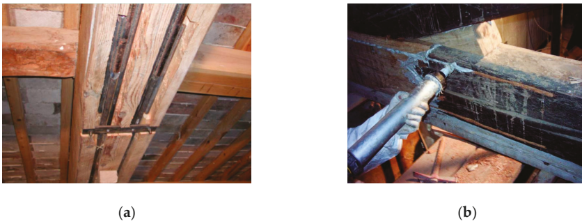
Figure 25. Bonded-in steel bar reinforcement: (a) detail of the reinforcement before resin application; (b) filling of the grooves with epoxy paste.
