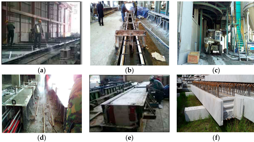
Figure 3. Production process of precast concrete girders (PCGs): (a) Spreading form oil; (b) rebar insert; (c) pouring concrete; (d) curing; (e) removal; (f) precast concrete girder.
