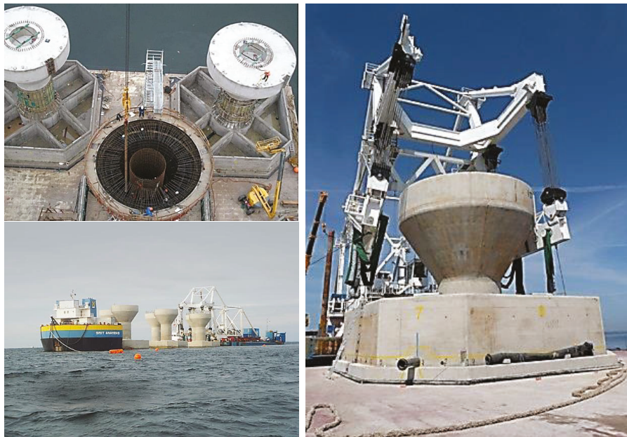
Figure 5. Rødsan II (or Nysted II) offshore wind farm foundations, reproduced from [22], with permission from Aarsleff, 2019.
