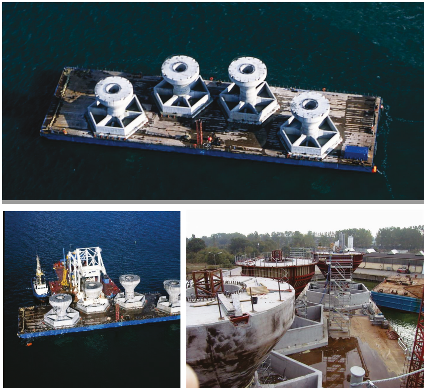
Figure 2. Nysted I (or Rødsan I) offshore wind farm foundations, with permission from Tech-Marine, 2019.
