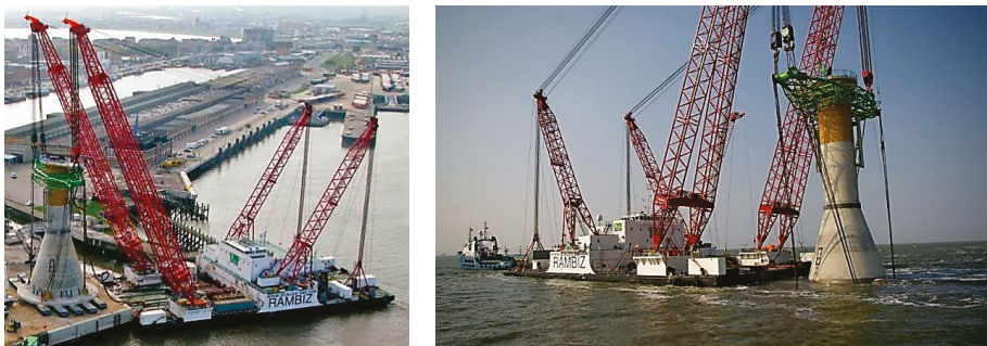
Figure 7. Thornton Bank offshore wind farm foundations, reproduced from [20], with permission from Elsevier, 2019.
