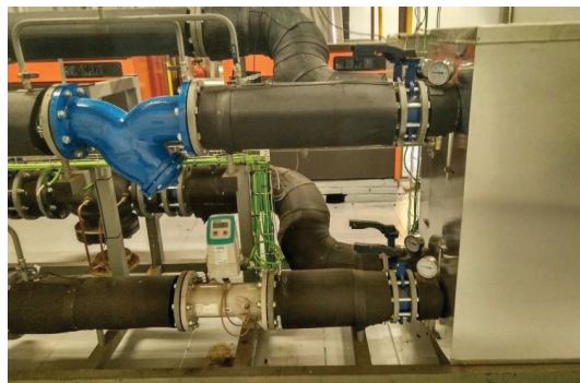
Figure 3. Heat exchanger substation in the facilities at the EII Building.
