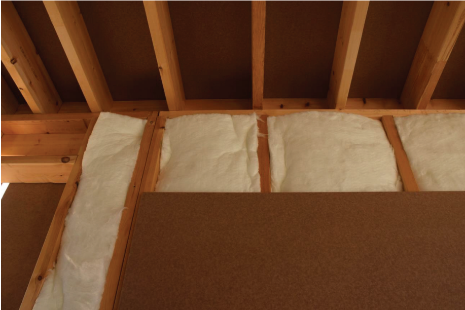
Figure 4. Wooden structure and Superpan Tech 15 mm board partitions with 148 mm mineral wool thermal insulation.
