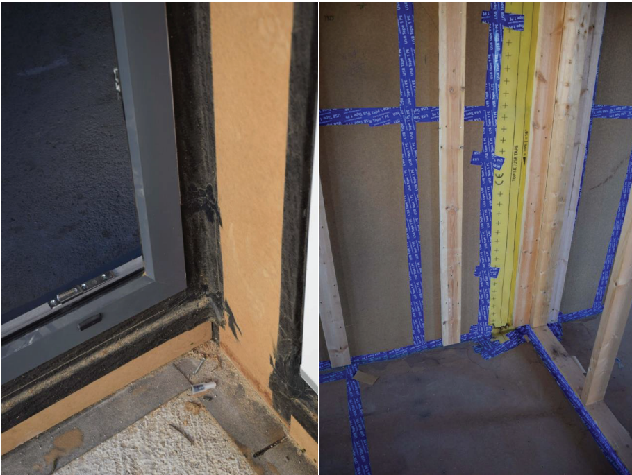
Figure 5. Lacquered aluminium carpentry joined to the exterior pavement. Airproof sealing and waterproofing with EPDM (left). Interior partitions and enclosure with tape sealing, type Riwega USB Tape 1 PE (right).
