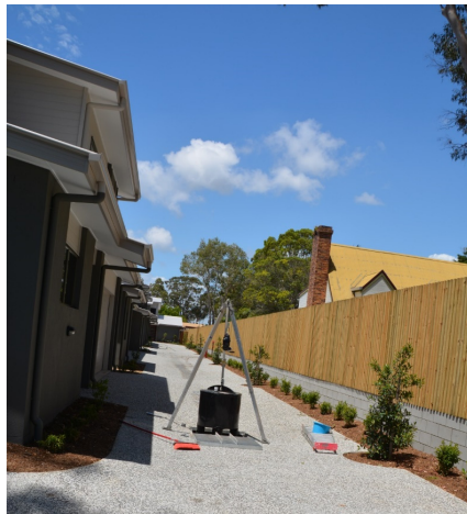
Figure 2. Townhouse development at Ormiston, QLD, showing driveway area, landscaping and filter cartridge for installation.
