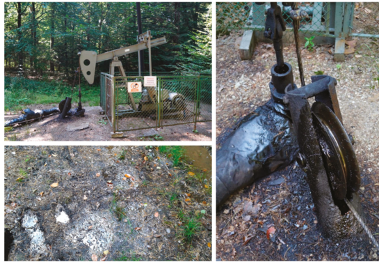
Figure 1. Sampling site of Bóbrka with spilled black crude oil.
