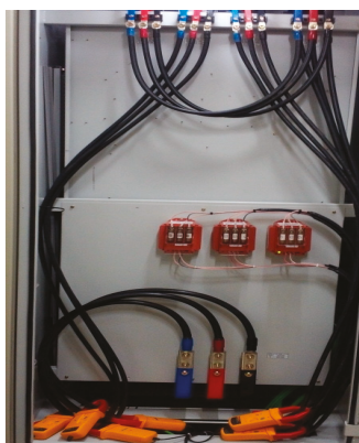
Figure 11. Installed voltage measuring equipment.
