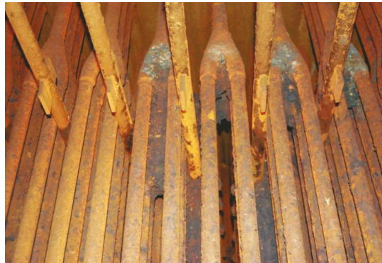
Figure 4. Tube bundle of the final steam superheater; an orange colouration is a distinctive feature of the accumulated corrosion layer. Grey and black deposits of flue gas components are highly visible between tubes.
