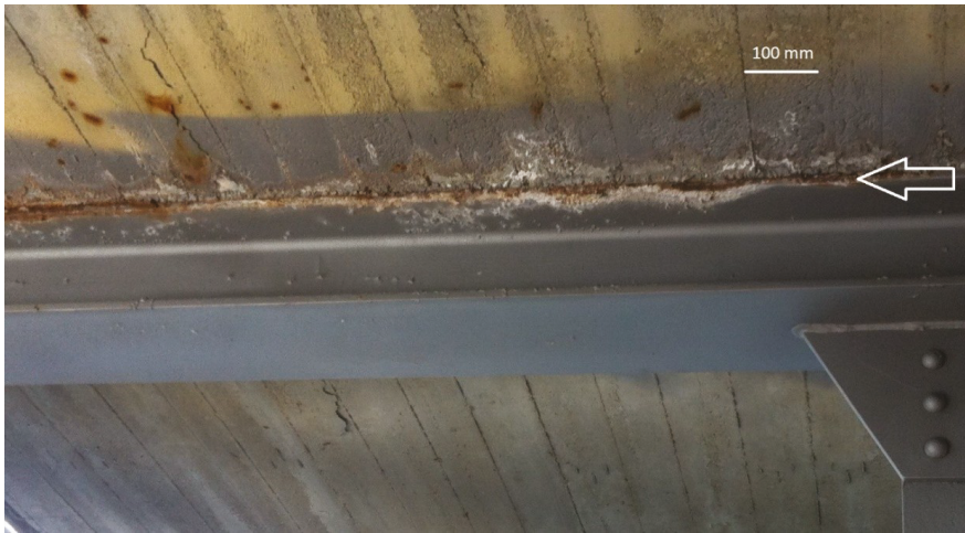
Figure 7. The saponification of alkyd paint where the painted H-beam is in contact with the concrete (marked with an arrow) and subsequent corrosion of zinc and steel.
