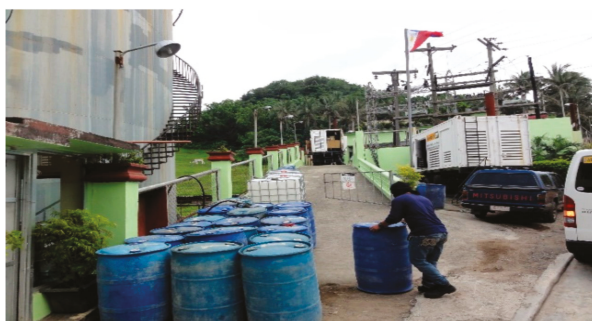
Figure 2. The Basco diesel power plant.
