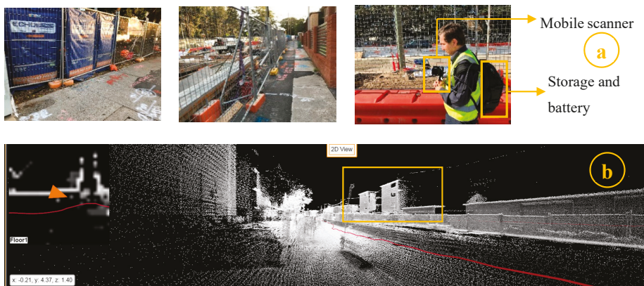
Figure 2. Infrastructure construction survey using a Geo SLAM (Simultaneous Localisation And Mapping) hand-held scanner: (a) data acquisition from a light rail project in Randwick, Sydney; (b) illustration of tracing route in red.
