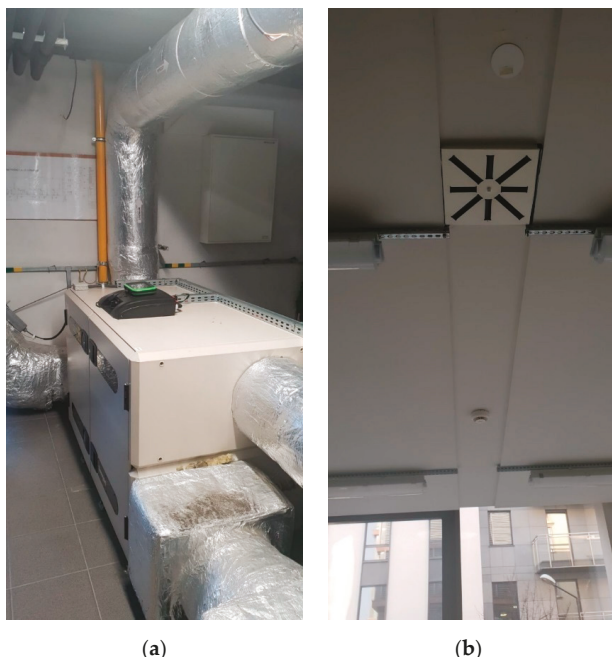
Figure 2. (a) View of the Air Handling Unit (AHU) with a recuperator with 90% efficiency. (b) The view of the intake vent grille in room P1.06; the grille is located in the central part of the ceiling.
