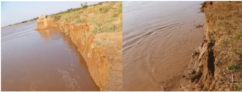
Figure 3. Example of the existing bank slope (left) and an example of riverbank collapse along Dengkou reach (right).
