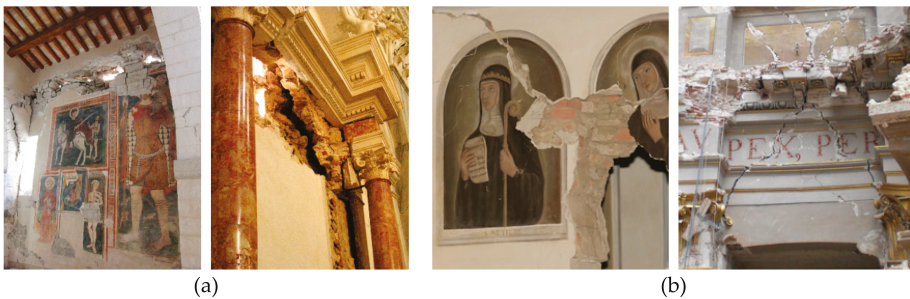
Figure 1. Examples of damage of artworks due to out-of-plane (a) and in-plane (b) mechanisms for frescoes and stuccoes.
