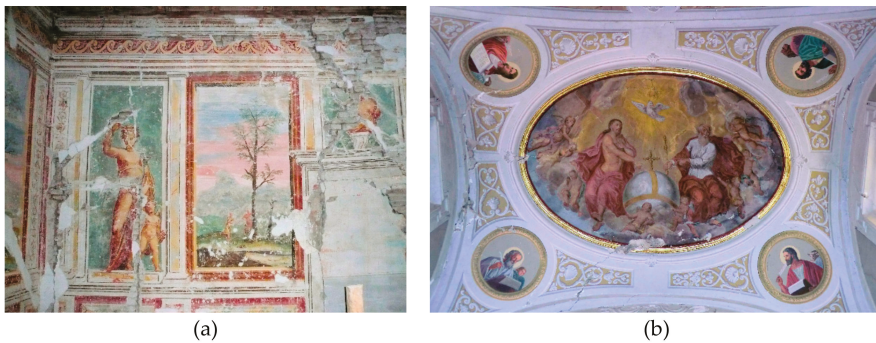
Figure 5. Example of primary and secondary mechanisms associated with a damaged fresco located in apse of a church: (a) apse is subjected to ‘overturning’, but the main mechanism affecting fresco is ‘shear’; therefore, ‘in-plane mechanism of apse’ and ‘overturning of apse’ are, respectively, primary and secondary mechanisms; (b) damage to the vault of the central nave affects the painting as a primary mechanism.
