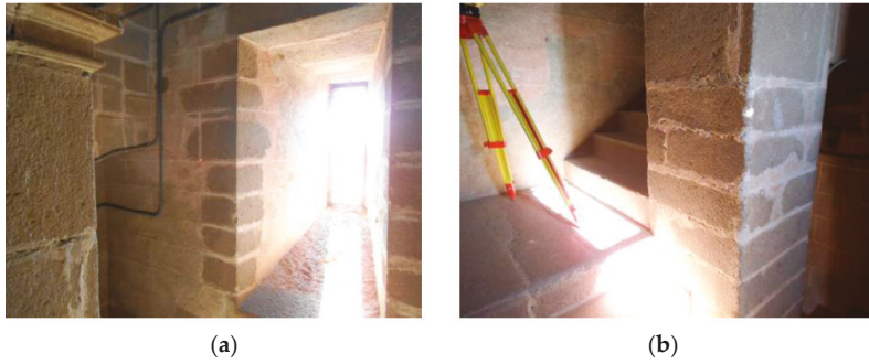
Figure 10. Walls built with granite ashlars (a,b). Interior of Santa María Church, Guareña (Spain).
