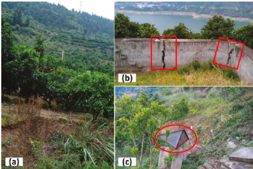
Figure 2. (a) Landscape of the landslide area; (b) Cracks on local infrastructure caused by the landslide; (c) one of the Corner Reflectors installed in the landslide area. Photos were taken during a field campaign in May 2014.
