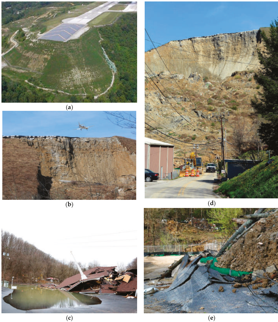
Figure 1. (a) Pre-failure photograph of the Yeager Airport [42]; (b) top of the landslide, showing the remains of the EMAS (white) and the geosynthetic reinforcements (Marcus Constantino, Charleston Gazette 12 March 2015 [44]); (c) the remains of the Keystone Apostolic Church, which was damaged by the landslide (Tyler Bell, Charleston Gazette 13 March 2015 [45]); (d) after the 2nd slope failure (F. Brian Ferguson, Charleston Gazette 13 April 2015 [46]); and (e) rolling up of asphalt at the toe of the landslide (Rusty Marks, Charleston Gazette 13 April 2015 [46]).
