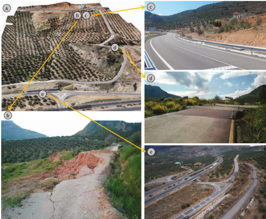
Figure 2. Landslide and affected roads: (a) Landslide general view; (b) Landslide head and the road JA-3200 interrupted; (c) Road JA-3200 after repair work; (d) Temporary road affected by an incipient unstable zone at the north of main landslide; (e) Landslide foot and affected access road to highway.
