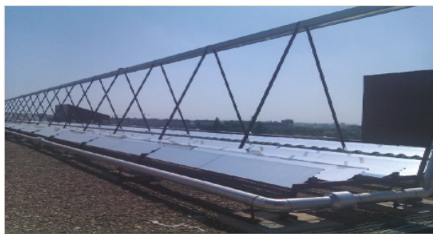
Figure 2. Fresnel collector field.
