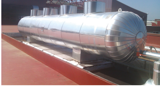
Figure 3. Phase change material (PCM) storage tank.
