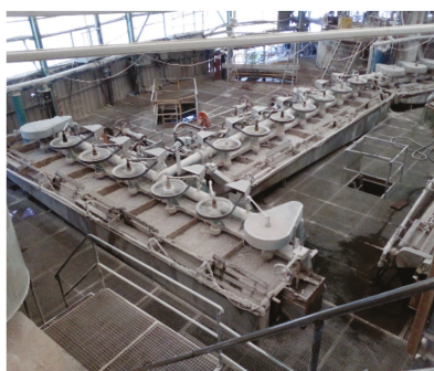
(a) Fluorite mine washing installations
