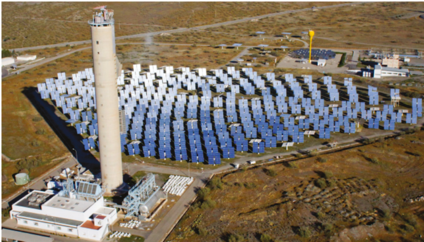
Figure 2. CSP heliostat field and solar tower at the Plataforma Solar de Almería, Spain (DLR).
