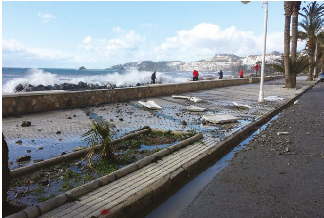
Figure 2. Severe damage after a western storm in winter 2015 at the Reina Sofia Promenade (Almuñecar), photo by europapress.
