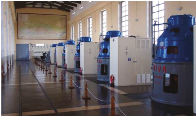
Figure 2. Hydraulic pumps in Mazzocchio’s pumping station.
