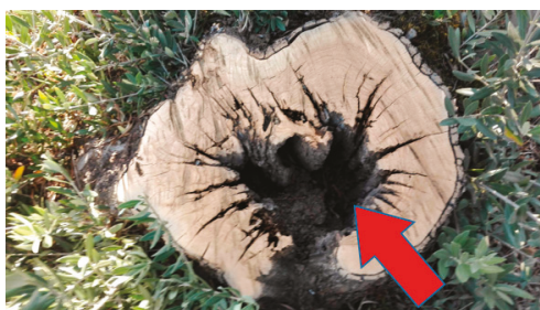
Figure 10. Felling the tree has shown the presence and size of the concealed damage (red arrow) detected by the IRT method.
