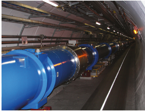
Figure 1. The LHC tunnel. The blue cryostat contains superconducting main dipole magnets. The protection unit is visible on the floor under the magnet (yellow rack). The photo taken by A.S. in 2007.
