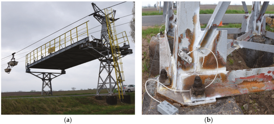
Figure 3. (a) View of column 1 with a safety platform. (b) View of anchor block and flanges at the connection between column 1 and foundation; signs of surface corrosion and pitting.
