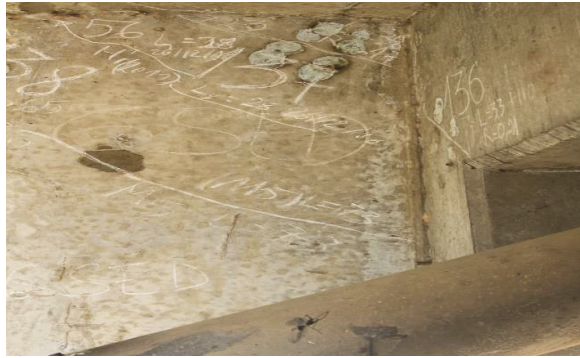
Figure 16. Examples of localized concrete cracks within the compression cables on My Thuan Bridge.
