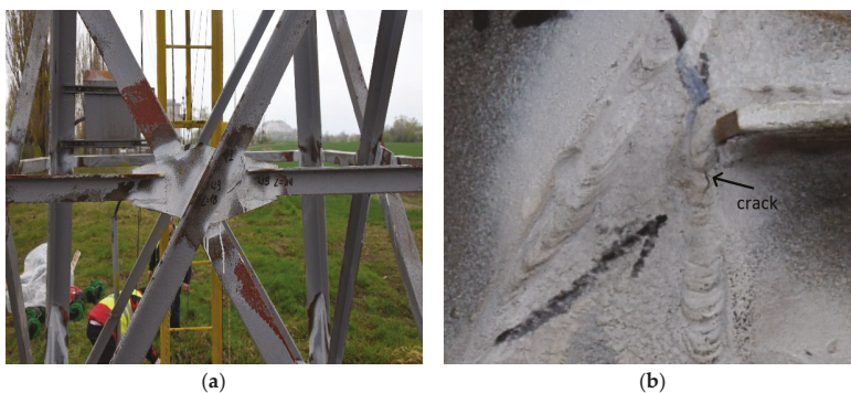
Figure 11. (a) Photograph of the tested node. on column 1 (b) A photograph of the crack detected on column 1.
