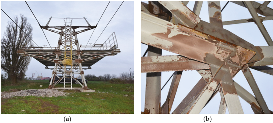
Figure 4. (a) Side view of column 2. (b) External view of the upper chord; signs of surface corrosion on truss members.
