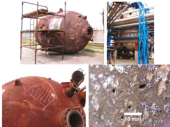
Figure 4. Breach of the cladding layer.
