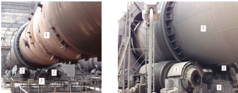
Figure 15. Rotary kiln on paired roller bearings. 1: kiln; 2: roller bearings; 3: support foundation.
