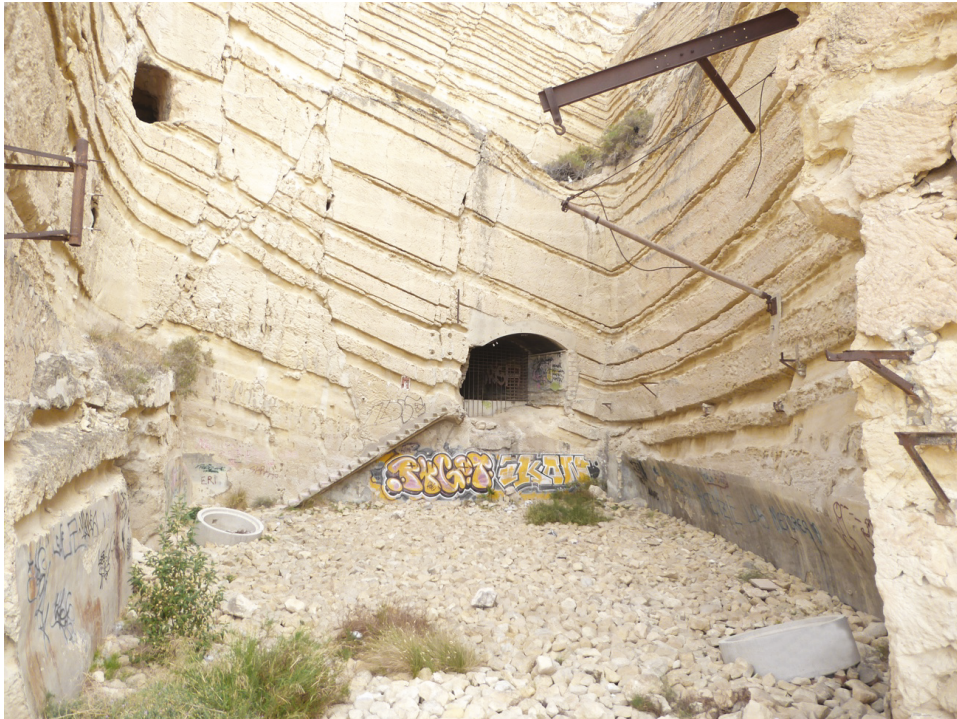
Figure 8. Image of the southern entrance to the complex, which was used as access to make the measurements taken from the stop of the TRAM de la Sangueta. It is trellised and in a deteriorated state such as the rest of the accesses (own source).
