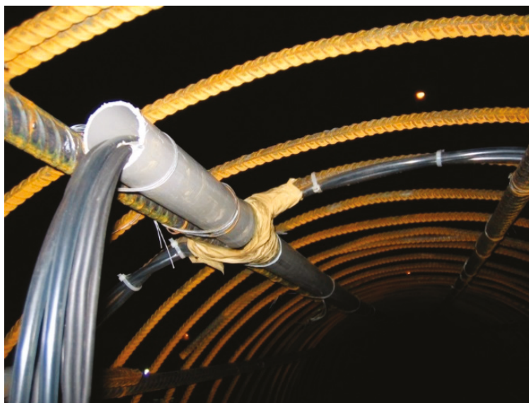
Figure 8. The electrical lead wires from the sensors come to the top.
