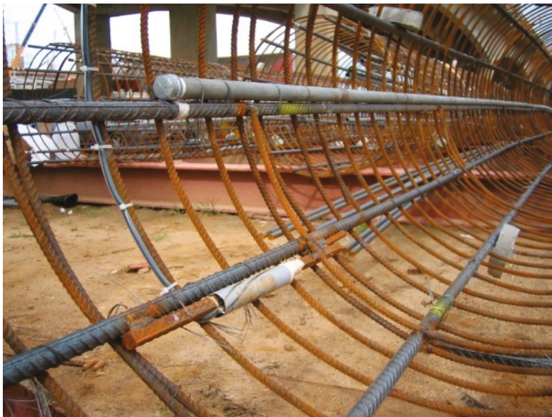
Figure 9. global strain extensometer pipe for tell-tales extensometer is pre-installed at VWSG.
