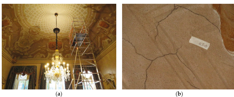
Figure 3. (a) Giunta room at Birago Palace; (b) cracks branched in the decorated plaster of the masonry vault in the Giunta room.
