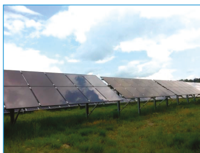
Figure 1. Experimental installation consisting of different PV (photovoltaic) module technologies.
