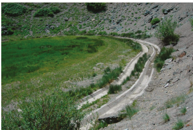
Figure 1. Mine spoil mitigation after installing soil cap that is protected from further contamination by stormwater runoff using collection and diversion channels.
