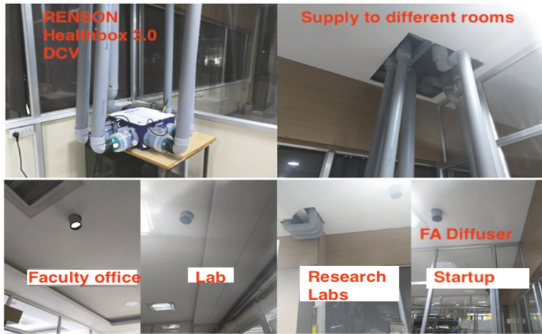
Figure 3. RENSON Healthbox 3.0 DCV Installation.
