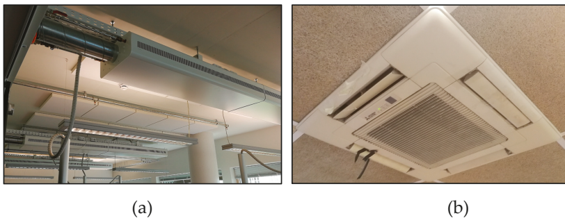
Figure 3. Possible air flow obstacles with open active beam solution (a); modified airflow distribution with fan coil unit (b).
