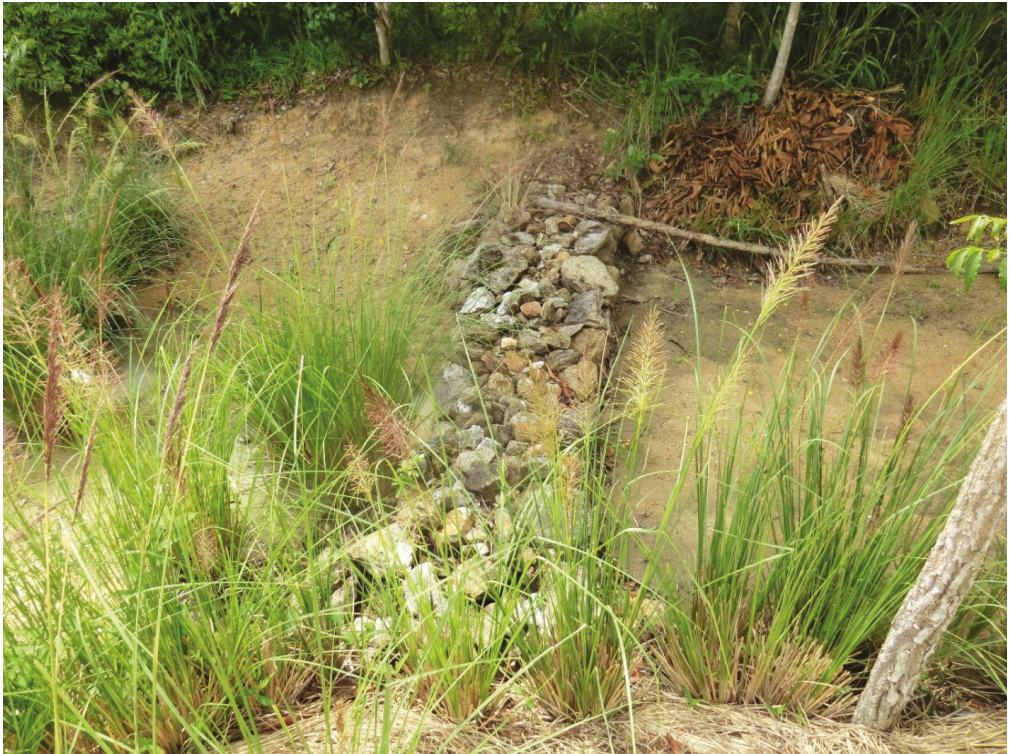
Figure 3. Erosion control measures including rock check dams and plantings of vetiver grass. Photo by Jonathan Long.
