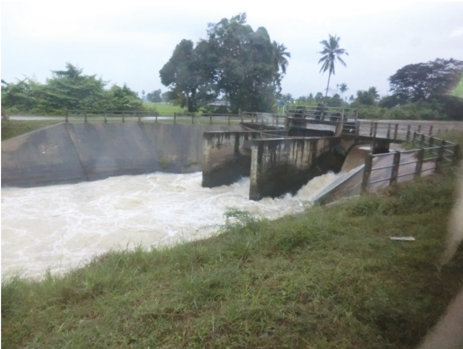
Figure 2. Water conveyance structure delivering water from storage reservoirs outside the SIEP watershed to downstream agriculture, cities, and tourism-related development. Photo by Jonathan Long.
