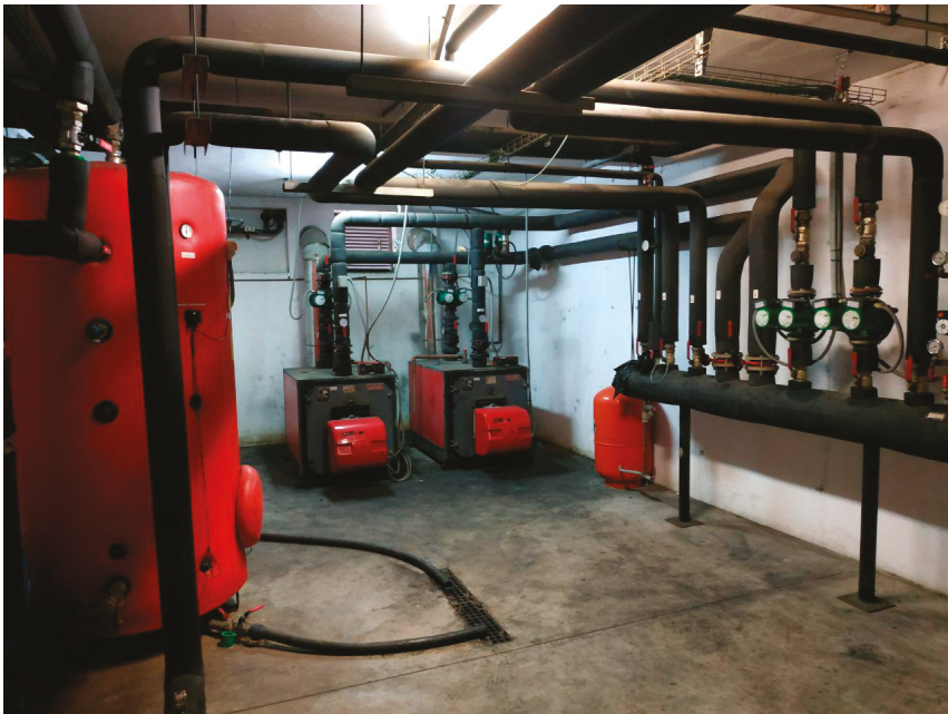
Figure 4. Boiler room of the indoor swimming pool.
