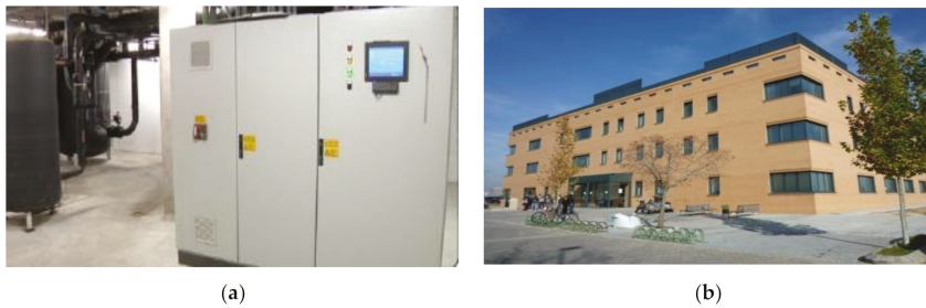
Figure 3. (a) Trigeneration Plant UAH's Polytechnic School; (b) UAH's Chemistry Faculty, a building of high efficiency due to the geothermal installation. © The University of Alcalá.
