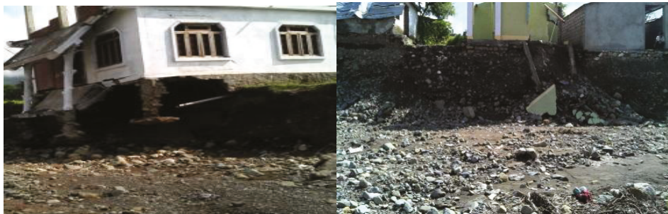
Figure 7. Affected infrastructures from the floods in the Itram River (photo taken by author, 2014).
