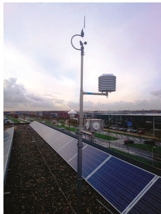
Figure 17. Weather station at the case study building.
