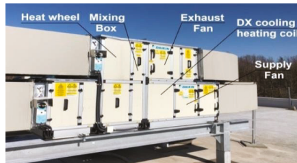
Figure 1. Photo from the investigated air handling units (AHU).
