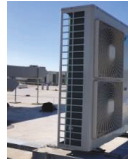
Figure 2. Photo from the outdoor unit.
