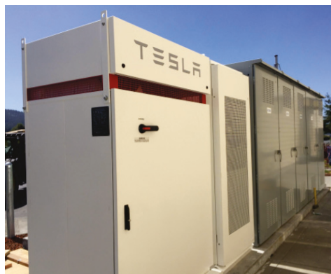
(b) 174 kWh local energy storage capacity with a peak output of 109 kW
