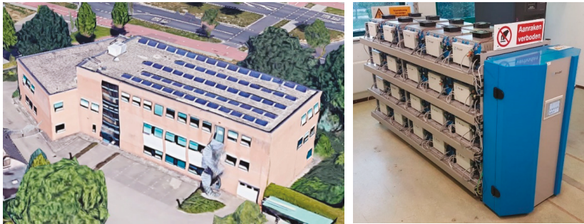
Figure 1. (Left) Impression of the building. (Right) A Battery Electric Storage System (BESS) installed inside the building.
