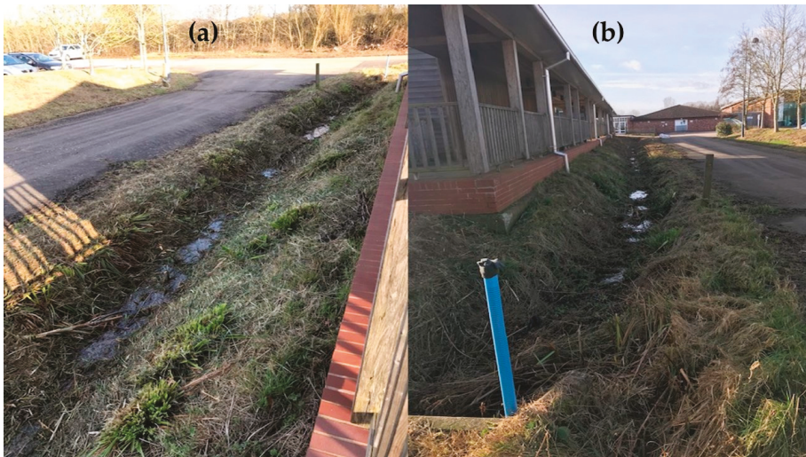
Figure 5. Detail of the swale after complete removal of vegetation (February 2020): (a) South-west sight of the swale; (b) North-east view of the swale from the discharge point and the monitoring device.
