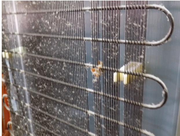
Figure 10. Typical fouling in a condenser.
