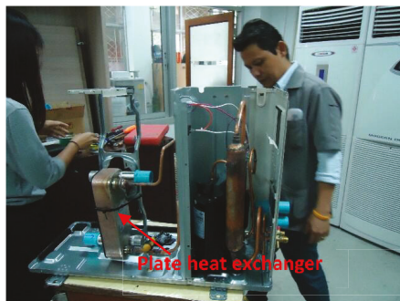
Figure 7. Modification of the air-source heat pump (ASHP) and installation of the plate heat exchanger.
