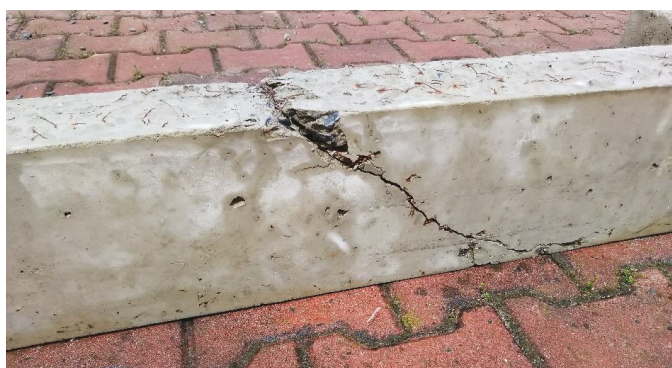
Figure 21. Details of a shear crack.
