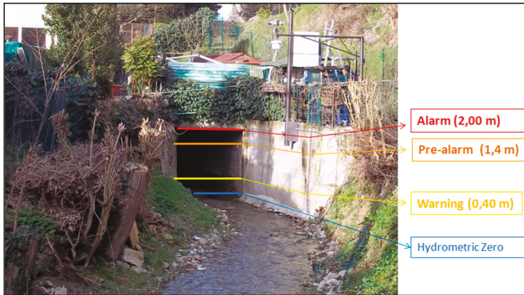
Figure 3. The entry of the culvert of the Ravone creek where the water level gauge is installed and the alarm thresholds are highlighted.
