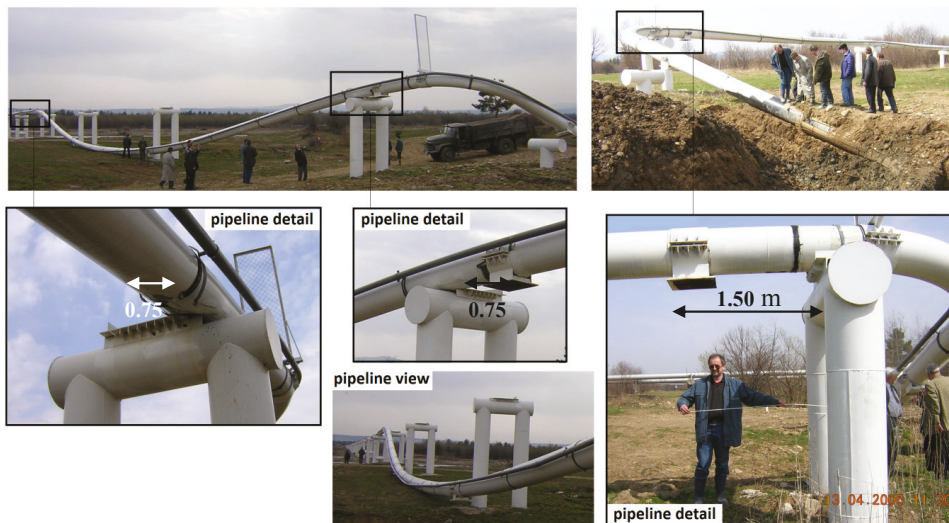
Figure 1. Pipeline accident (adapted from [23]).
