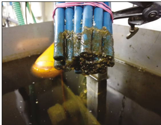
Figure 16. The sensor array after long-term online measurements at an aeration water plant. The sensors were cleaned by intensive washing. In spite of significant contamination, the sensors were stable for at least two months [79].
